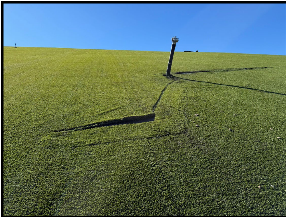
Photograph 6: View of additional damage related to DTC-1 on north side of Area 1-2.
