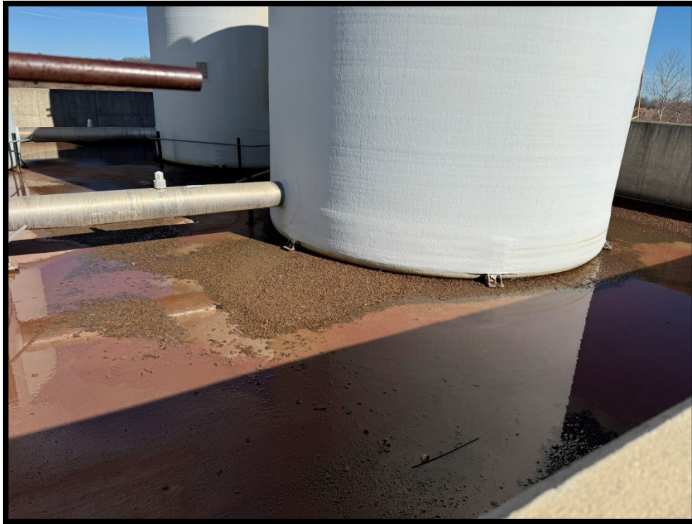
Photograph 3: View of minimal stormwater in leachate tank containment.
