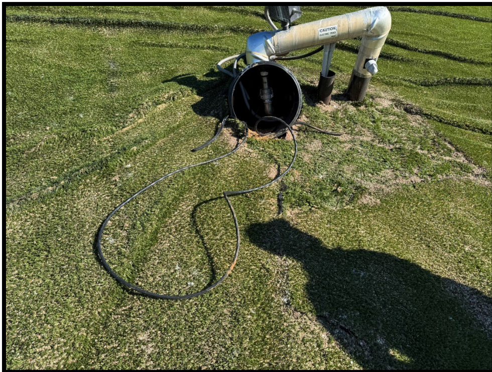
Photograph 4: View of wire trace and wooden cover removed from LCS-4 sump housing.
