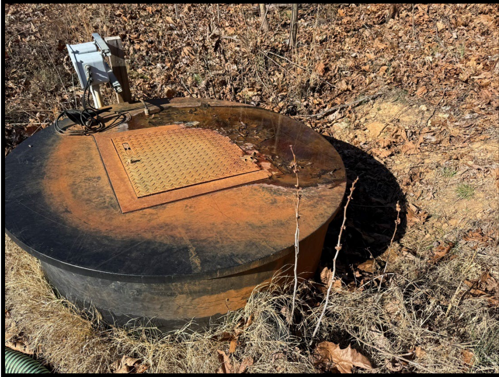
Photograph 1: View of VLCS-1 overflowing.
